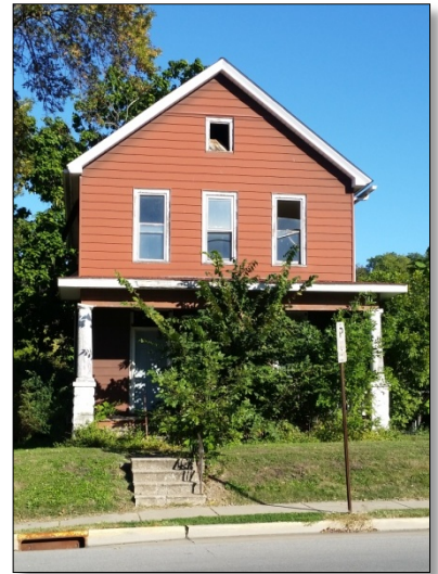
This abandoned single family home was recently purchased by the City via the annual county tax sale; it is slated to be demolished due to neglect.
